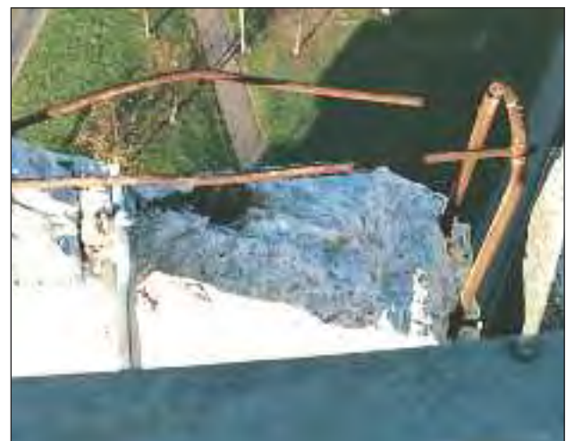
Lightning strikes can cause major structural damage to buildings
