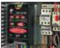
ESP 415 M1 installed within a control panel on the mains input to protect the panel's control systems. Note the remote indication connection (top of protector)
